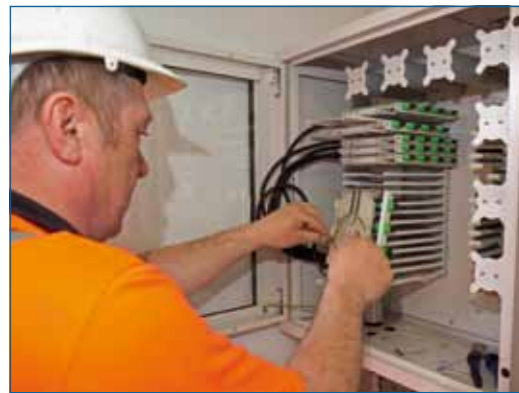
FTN / GSM-R Power Connections Client: Network Rail Date: August 2011 - ongoing
