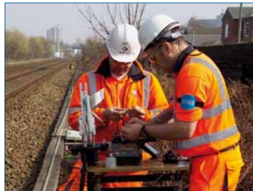
FTN / GSM-R Fibre and Copper Tails Framework Client: Network Rail Date: January 2011 - ongoing
