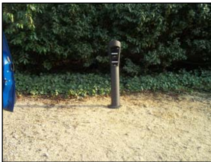
Electric Vehicle Charging Point (EVCP)
